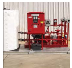
Diesel Pump Skids
